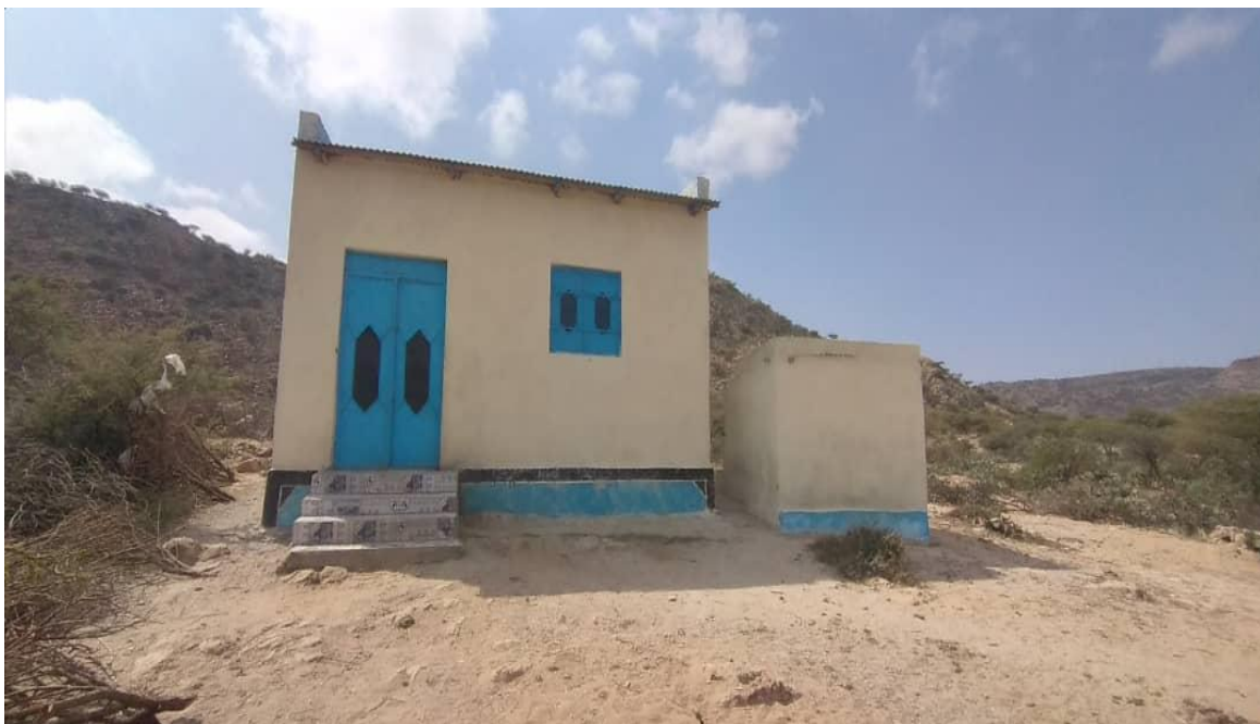
Construction of a security room and Construction of a latrine for visitors
